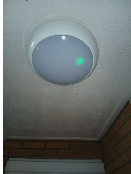
Lighting (Standard and Emergency Lights)
